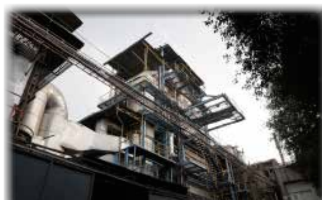
Co-Gen plant for Turbine Generator MIL unit-1 Hapur
