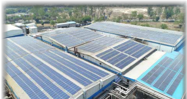
Solar Panels on rooftops of factory in Hapur
