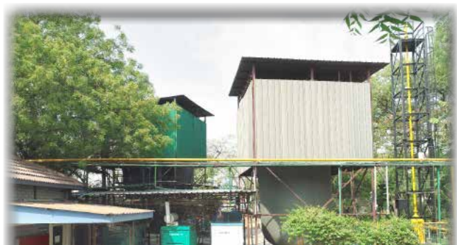
Bio Gas plant in MIL unit-1
